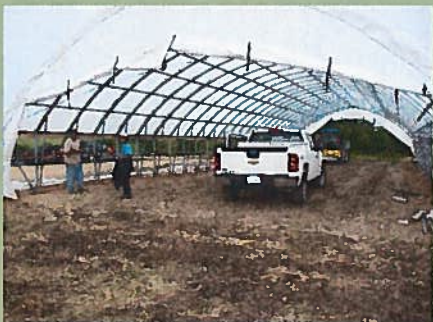
NRCS provided funding support to assist agricultural producers in the county to install, "High Tunnel" houses for growing vegetables and berries.
