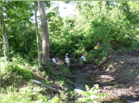
Workers collect debris at the NRCS' Collinsville EWP site.
